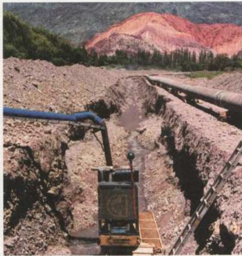
Excavating a ditch for the pipeline in Rio Purmamarca. The riverbed was restored and steps were taken to protect the small irrigation systems of local farmers.
