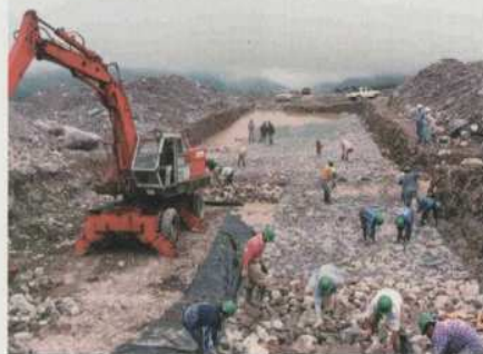
Top: the pipeline passes through narrow and steep rights-of-way through the mountains. Above: local labourers help place a 57-metre, one-metre thick gabion mat over the pipeline as protection.
