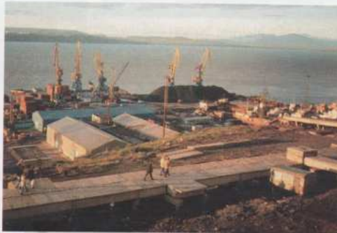
FSC is back in Russia for construction of an arena and a hangar in Anadyr, the Chukotka capital.
